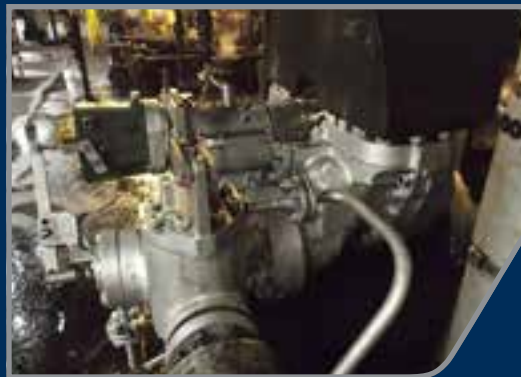
With Steam Turbine Seal.
