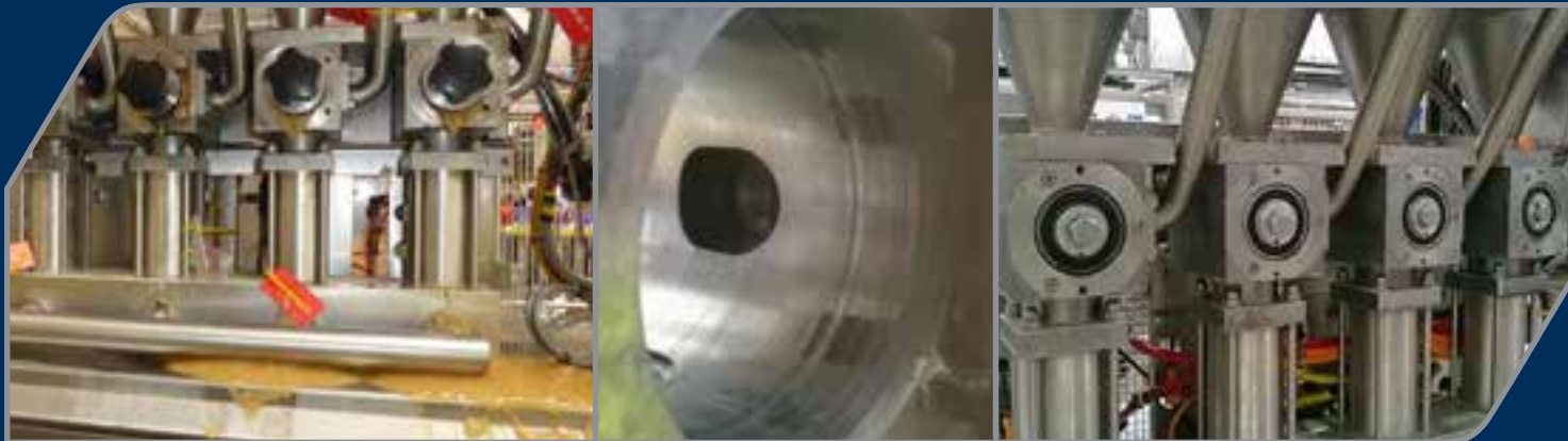
Line before upgrade — product leakage clearly seen.
