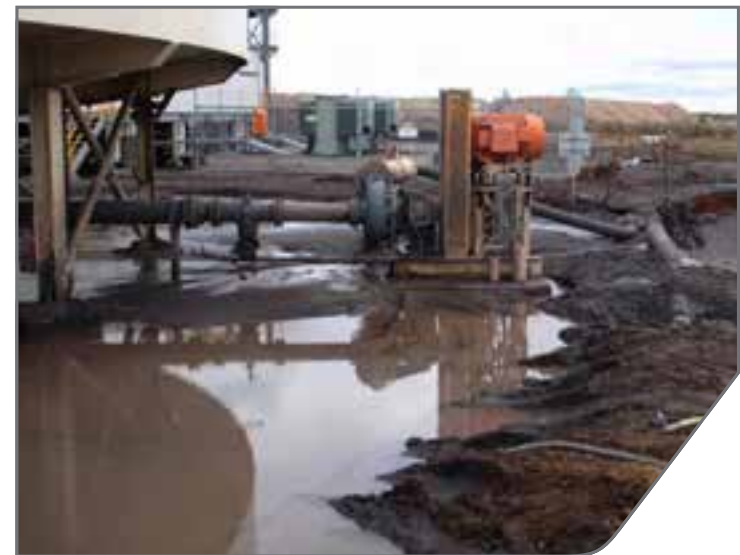
Typical mining slurry pump with packing gland water can create a safety hazard and waste water.
